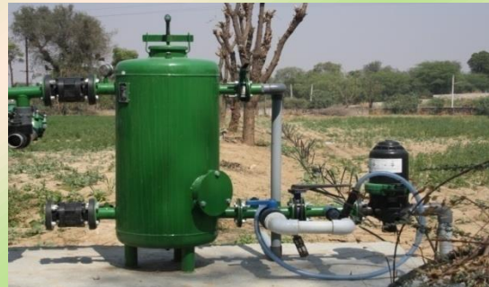
Drip irrigation system installed at SKNCOA, Jobner
