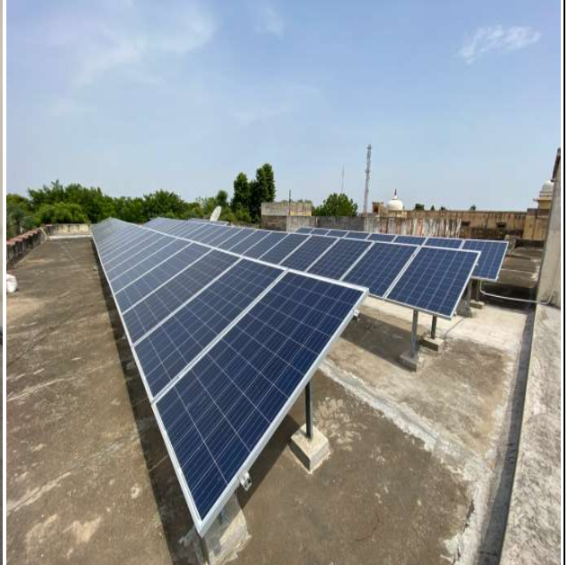
Solar plate Installed at University Building
